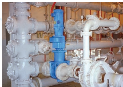
A SUPER SHREDDER in a sludge re-circulation line.
